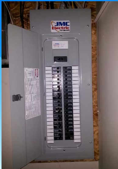
200 Amp Electrical Panel
